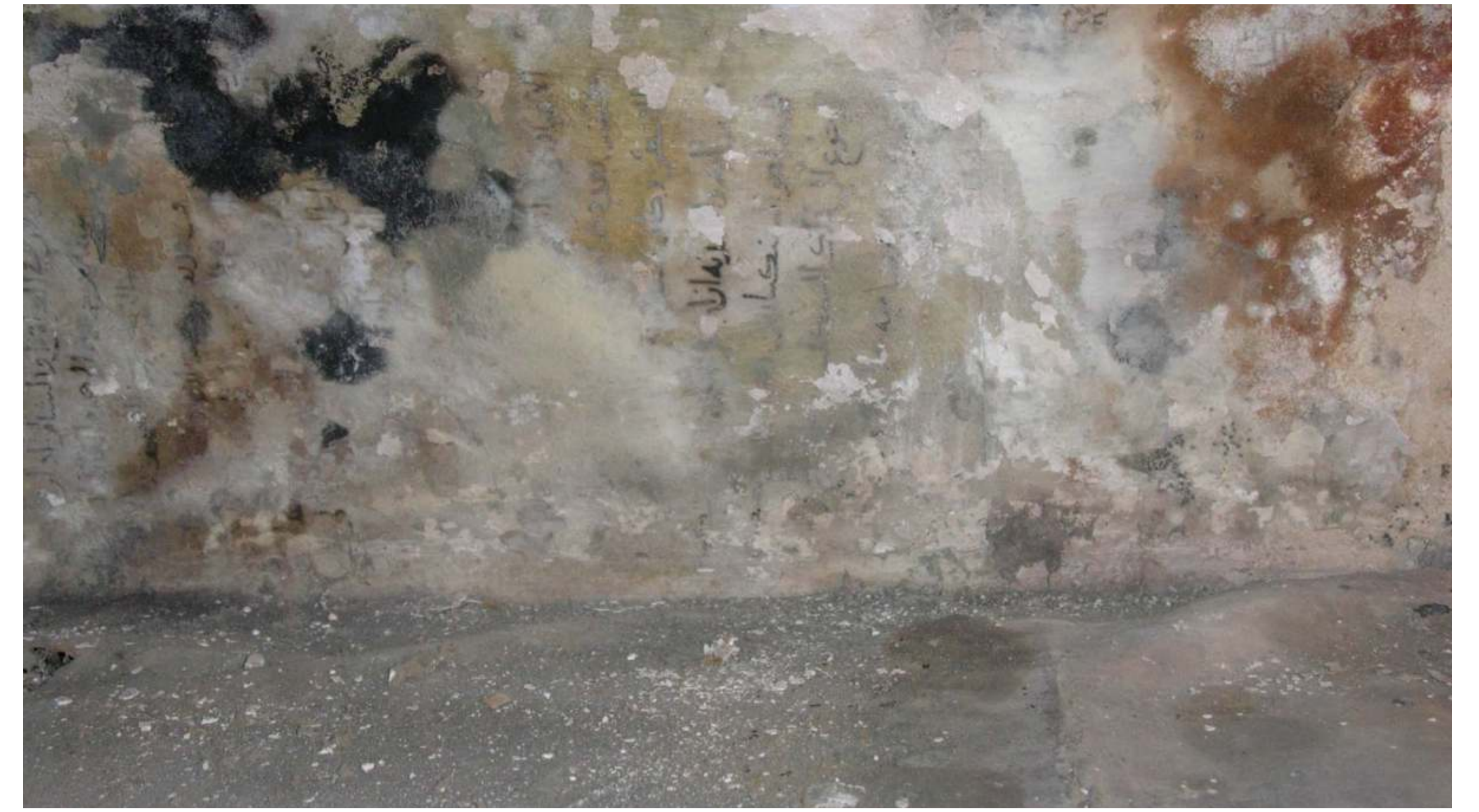
The upper level of fragments showing the extensive mould growth.
